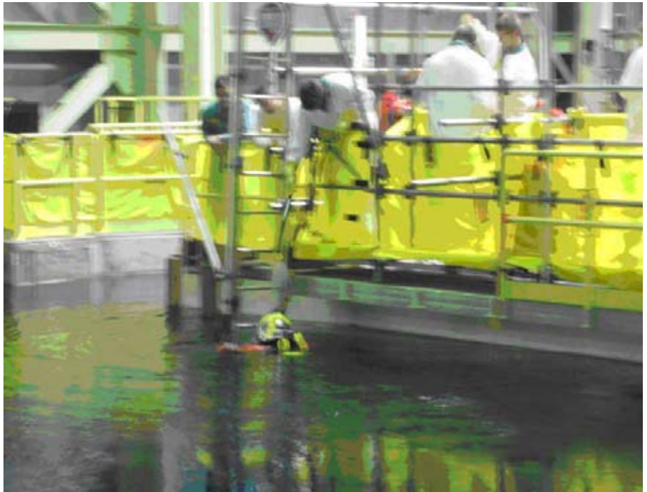
ASI Group diver Dave Reaker entered the secondary irradiated fuel bay (SIFB) to make liner repairs. This is the first time in Canada a dive has been made into a bay containing irradiated fuel.
